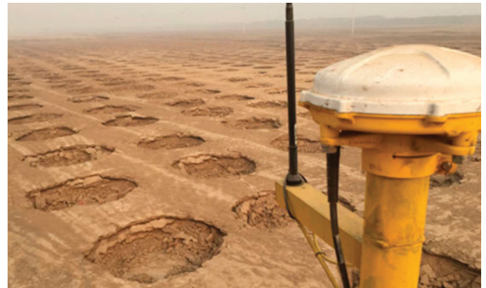
Accurate spacing between hammer drops was critical, but with a GNSS on-machine guidance system the compaction team easily achieved the accuracy they needed without stakes.
